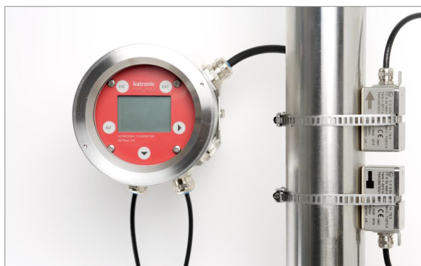
KATflow 170 in operation
