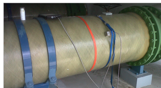
KATflow 230 and K0 transducers installed on large fiberglass pipe
