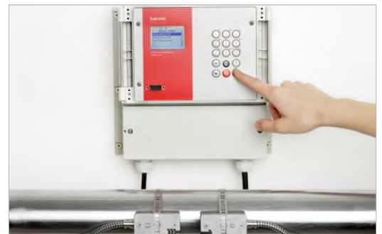
The fixed clamp-on flowmeter KATflow 150 provided reliable flow data to the German water supplier.
